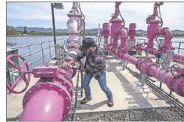
Billy Dixon, engineering technician with Sonoma Water, closes a valve April 29 at the new recycled water reservoir
